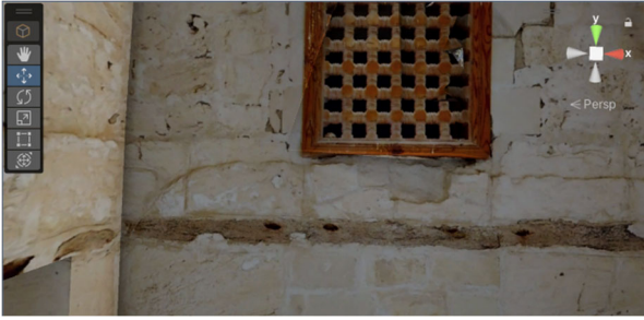
Figure 19: Deterioration in the wooden tie beam in Matterport model on Unity Platform.
